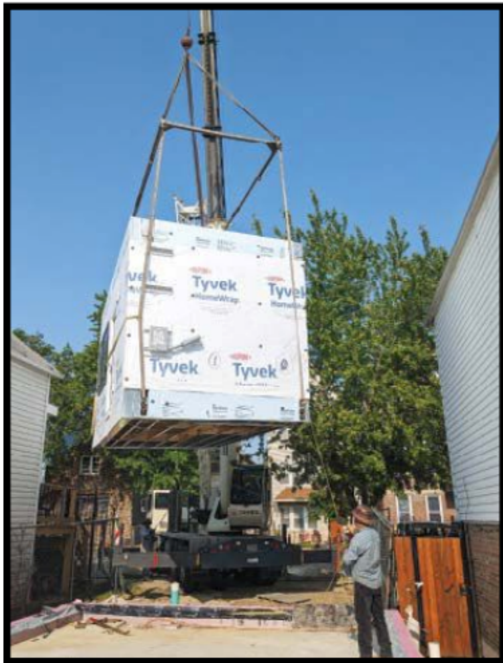
Space-constrained sites, like this one in Chicago, create challenges for crane operators placing modules.
